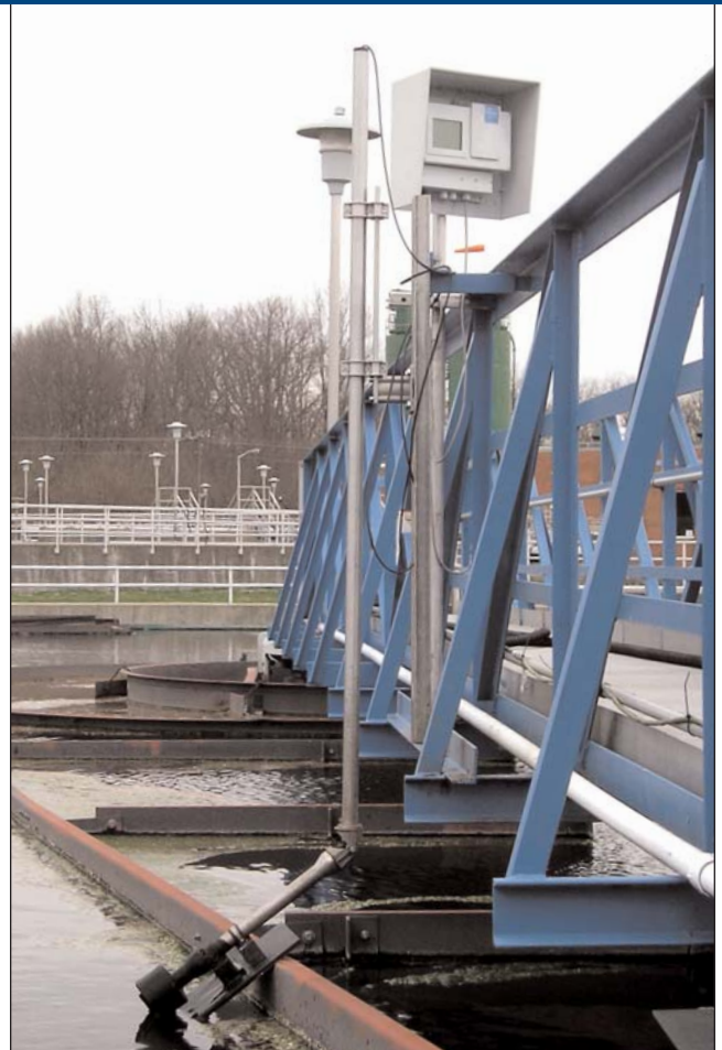
An on-line Hach Sludge Blanket Level Monitor with graphic display helps West Hickman Creek WWTP operators control sludge pumping to minimize phosphorus in final clarifier effluent. The sensor is mounted on a three-foot pivot for convenient retrieval.
